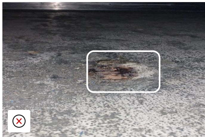
Resin floor protective coat holed & floor board beneath exposed
