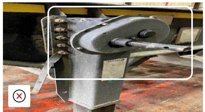
Winding handle missing and needs to be replaced
