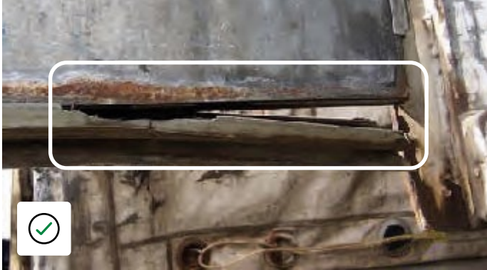
Old door with corrosion to inner skin, damage to seals due to continuous use no distortion to door panel.
