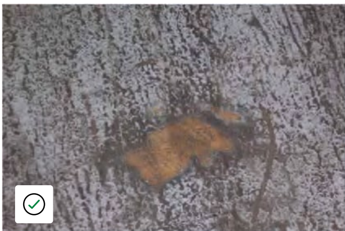
Resin floor top protective coat worn
