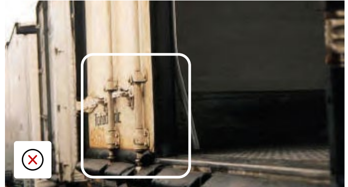
Damaged door seal aluminium trim.
