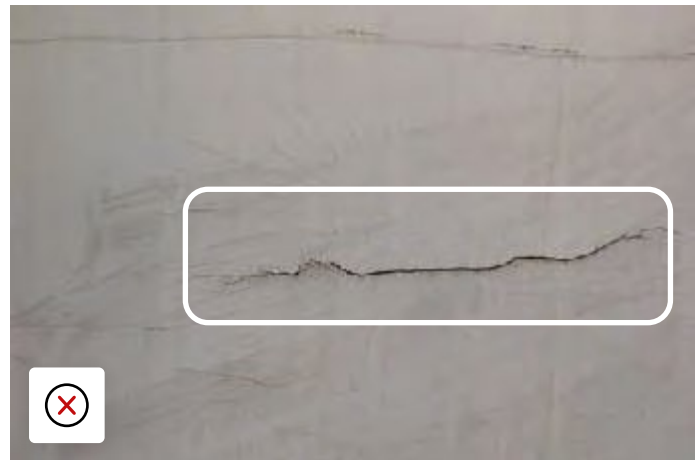
GRP side panel crack with water ingress, fine cracks indicate interior impact.
