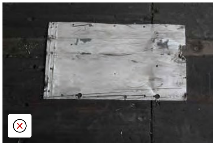
Metal plate over damaged floor section.
