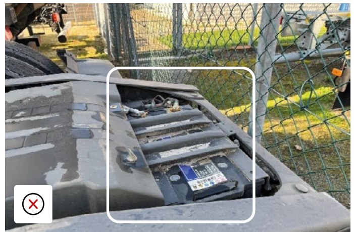
Battery cover missing - exposing battery to the elements
