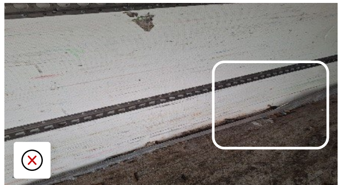
Kick strip damaged and pulled away from panel.
