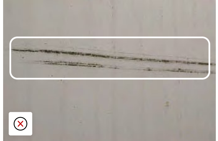
GRP side panel scrape Gelcoat coating broken, water ingress and now mildew infection
