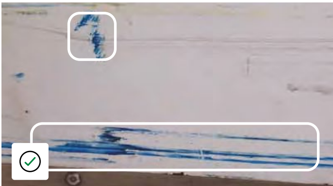
GRP panel scraped by pallets but not penetrating Gelcoat.
