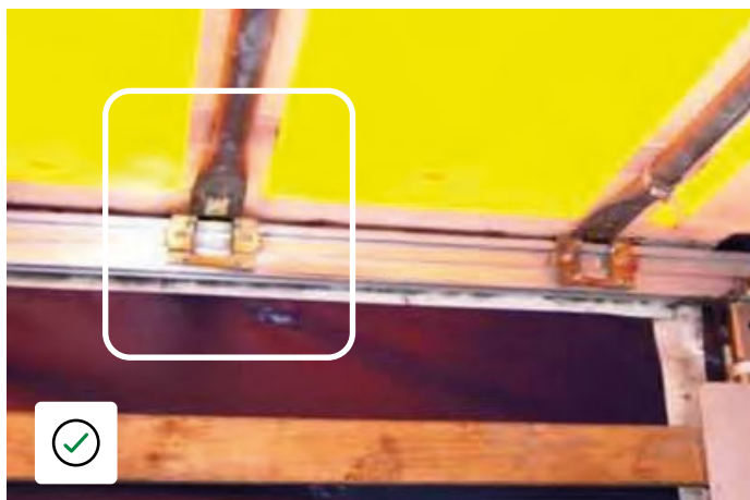
Edscha roof with securing strap missing, no sign of damage, strap is wear item.
