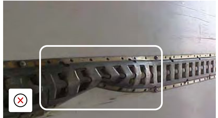
Interior load control damaged beyond repair.
