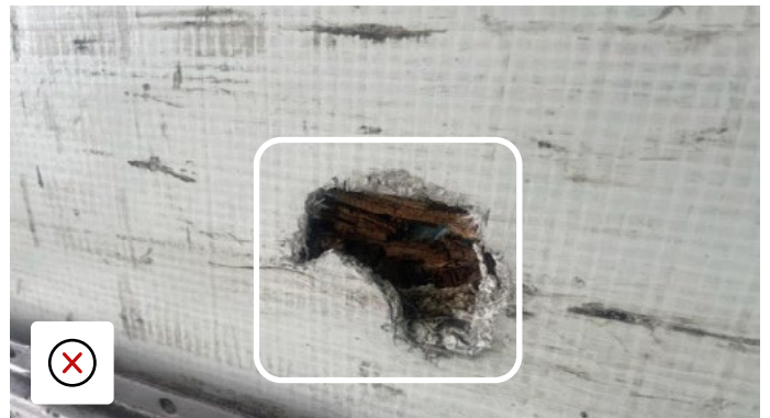
GRP panel penetrated & wood exposed
