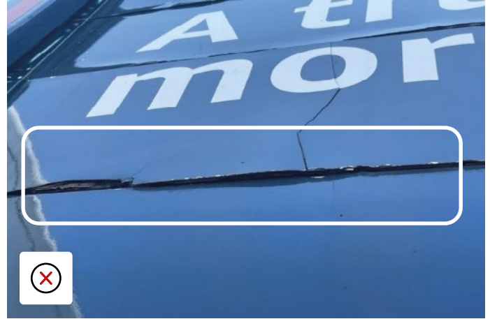
Door panel on roll shutter cracked due to impact
