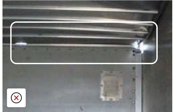
Damage to front roof sheet
