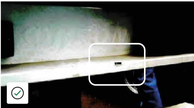
Impact damage that does not distort the Fabrication and can be cleaned and painted at little expense.
