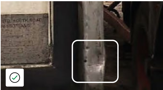
Bent rear door hinge support due to impact, not impairing the door operation.
