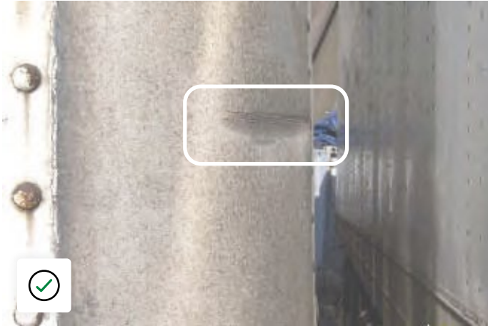
Corner post damaged due to impact dented but not holed.
