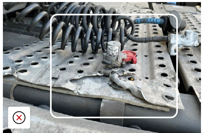
Catwalk damaged causing trip hazard
