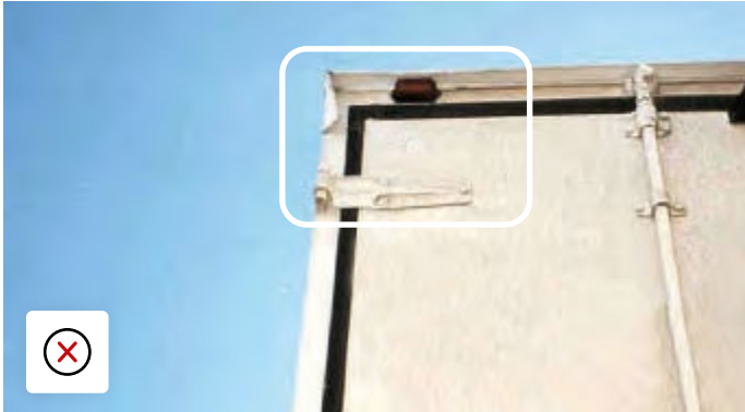
Bent rear door frame water protection trims due to impact.
